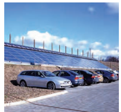
Solar panel roof of the crop store integrated with landscaping at the Renewable Energy Centre, Hertfordshire.
