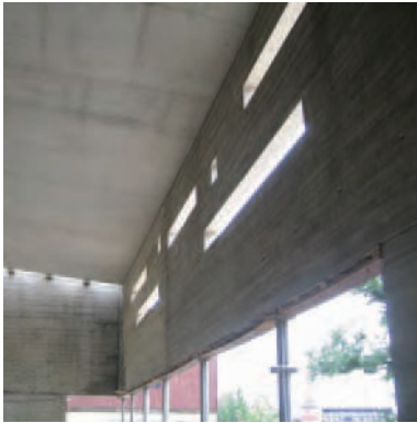
The café wall with 7 openings built in one pour using self-compacting concrete at the City & County Museum, Lincoln.
